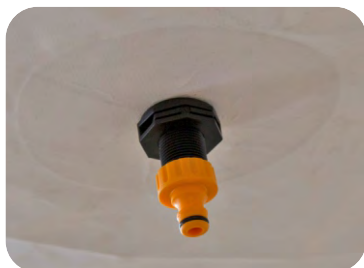
Central Drainage Point
